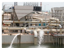
Water Treatment Facility
